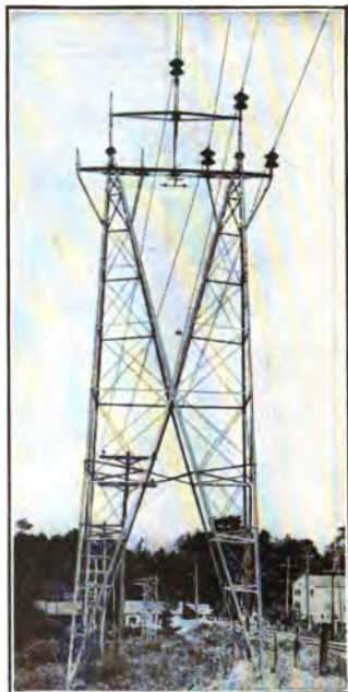
FIG. 57.—Double circuit three-phase steel tower, 50 feet high, for 66,000 volts.
