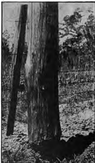
FIG. 353.—Untreated chestnut pole decayed at ground line.
