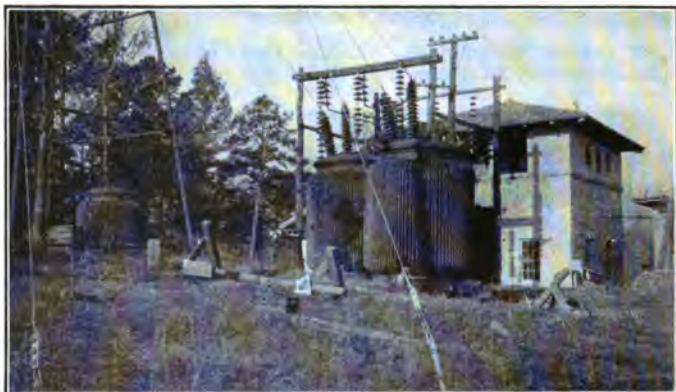
FIG. 66.—Outdoor sub-station, three-phase 3-2000 kv-a transformers, 101,100 volts to 13,200 volts, 60 cycles.
