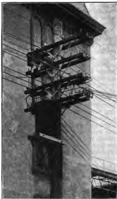
FIG. 395.—Individual transformer installation.
