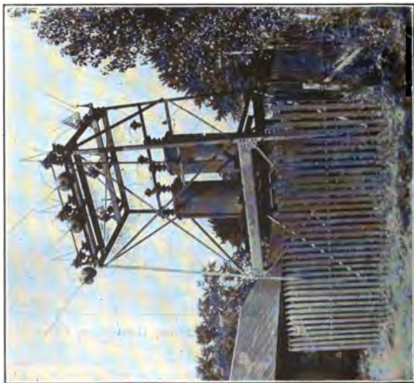
Fig. 70.—Outdoor sub-station, three-phase 2-50 kv-a, 33,000/12,300 volt, 60 cycle transformers.
