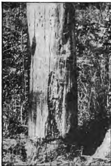
Fig. 350.—Untreated cedar pole decayed at ground line and upward about two feet.
