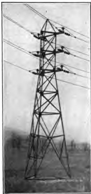
FIG. 58.—Double circuit steel corner tower, 40 feet high.
