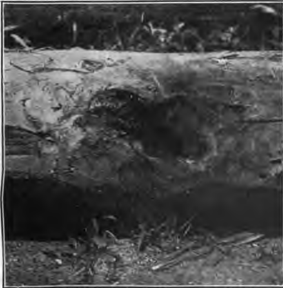
Fig. 23.—Hollow Knot indicating Heart Rot in Eastern White Cedar Pole.
