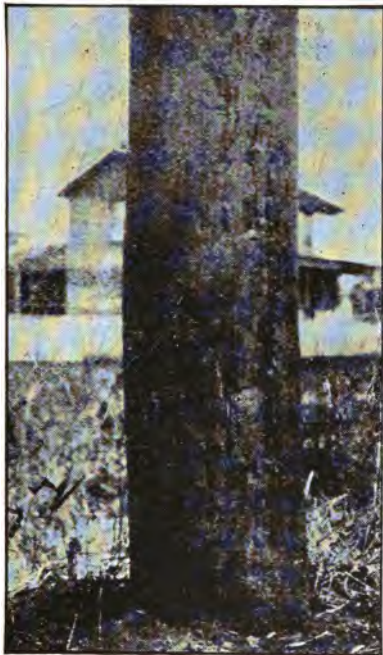
FIG. 354.—Pressure creosoted pine pole—18 years' service under southern climatic conditions. No decay to date.
