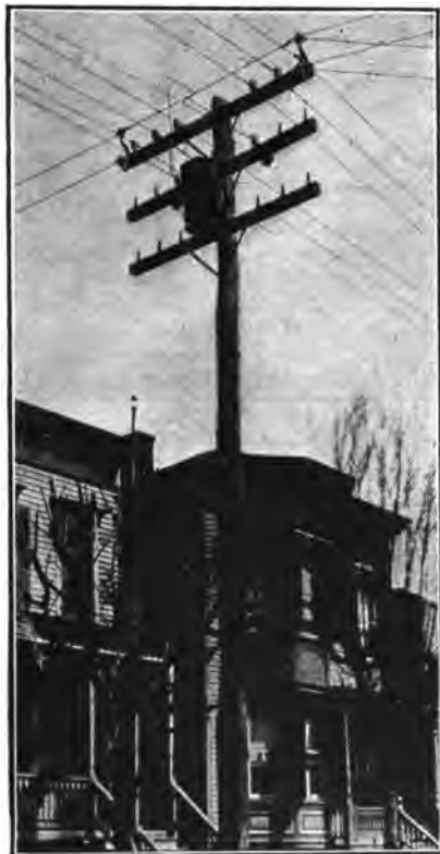
FIG. 396.—Individual transformer installation.
