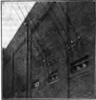
FIG. 421.—Line entrance bushings. (Sub-station.)
