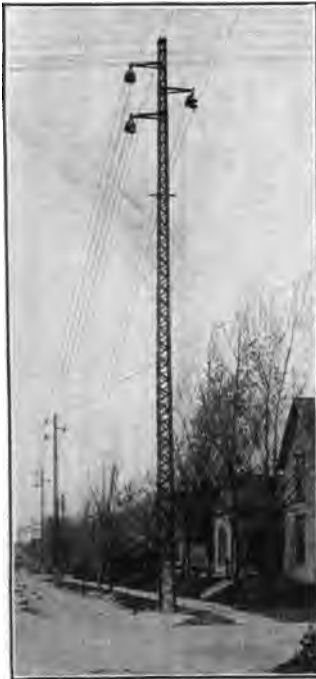
FIG. 45.—Single circuit three-phase 30,000 volt steel pole.
