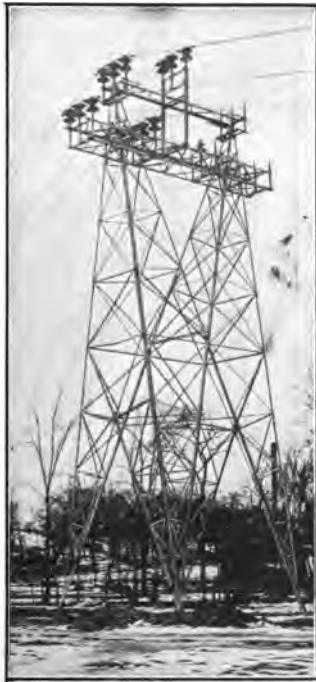
FIG. 63.—Double circuit three-phase steel corner tower, 50 feet high, for 66,000 volts.
