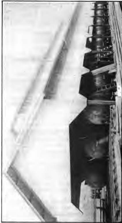
FIG. 345.—View of pressure treating cylinders.
