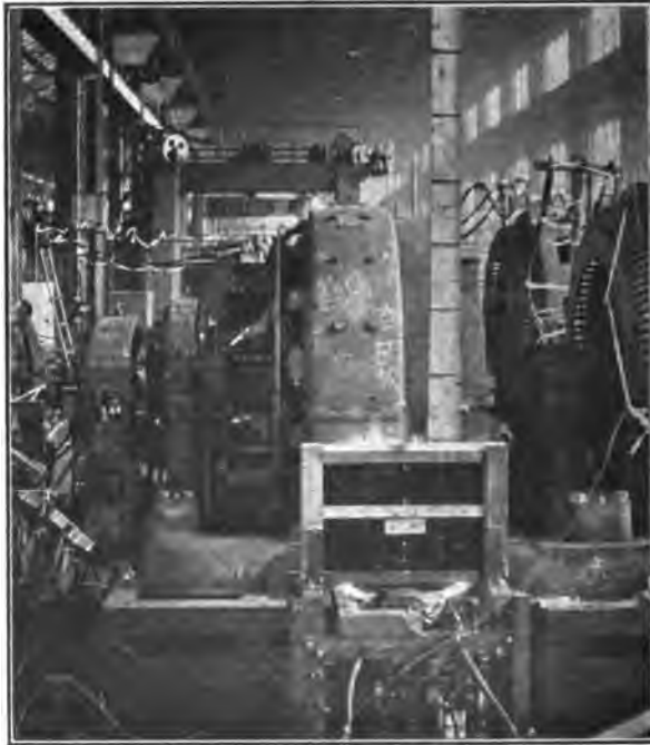
FIG. 4—SHORT CIRCUIT ON 2000-Kw., 3000-VOLT MOTOR-GENERATOR SET PROTECTED BY HIGH-SPEED CIRCUIT BREAKER AND FLASH BARRIERS. TRIPPING POINT 2550 AMPERES. LINE RESISTANCE 0. CURRENT LIMITING RESISTANCE 1.2 OHMS
