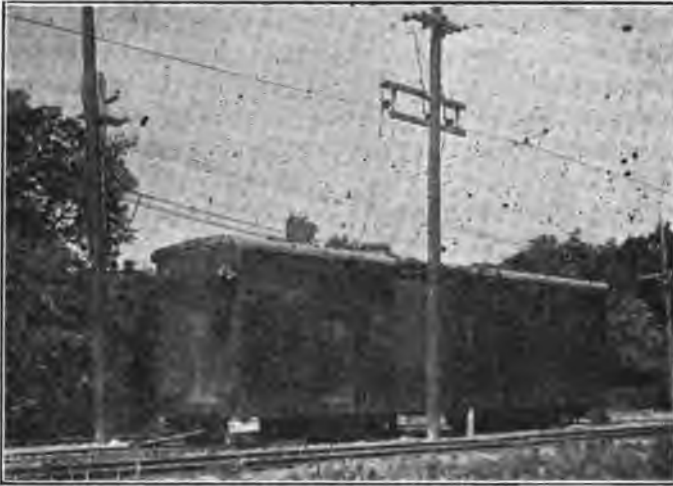
FIG. 6—PORTABLE AUTOMATIC SUBSTATION CONTAINING 500-Kw. 600-VOLT SYNCHRONOUS CONVERTER—KANSAS CITY RAILWAYS Co.
