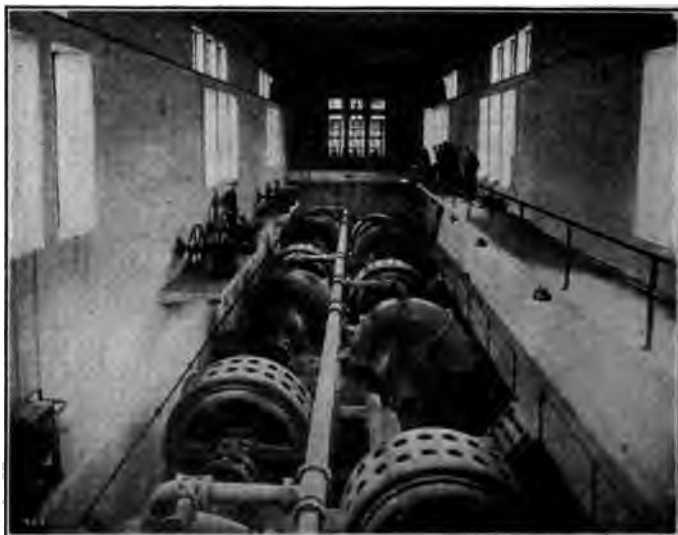
FIG. 5 INTERIOR VIEW OF PUMPING PLANT
