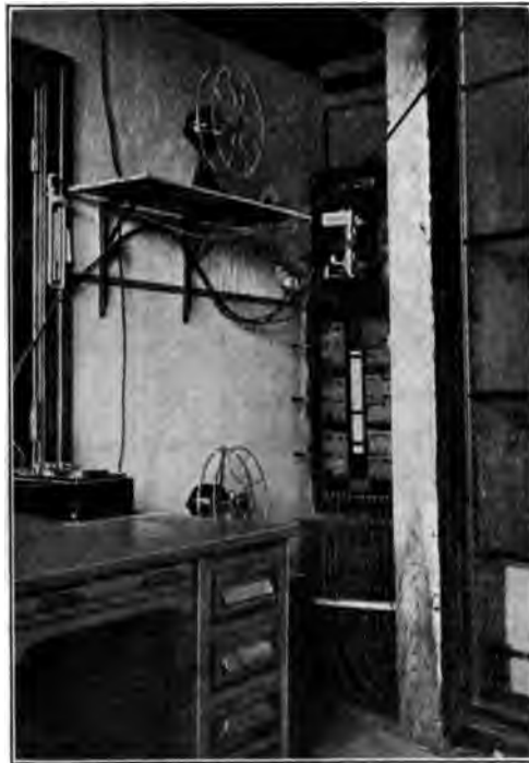
FIG. 3 GENERAL ARRANGEMENT OF APPARATUS, SHOWING FANS, SWITCHBOARDS, METERS, ETC.
