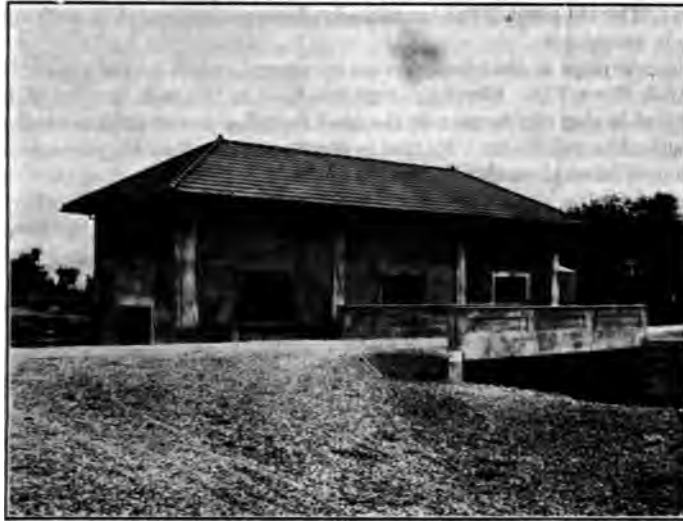
FIG. 26 PUMPING PLANT, CITRUS, LA., SHOWING DISCHARGE SIDE FACING LAKE PONTCHARTRAIN
