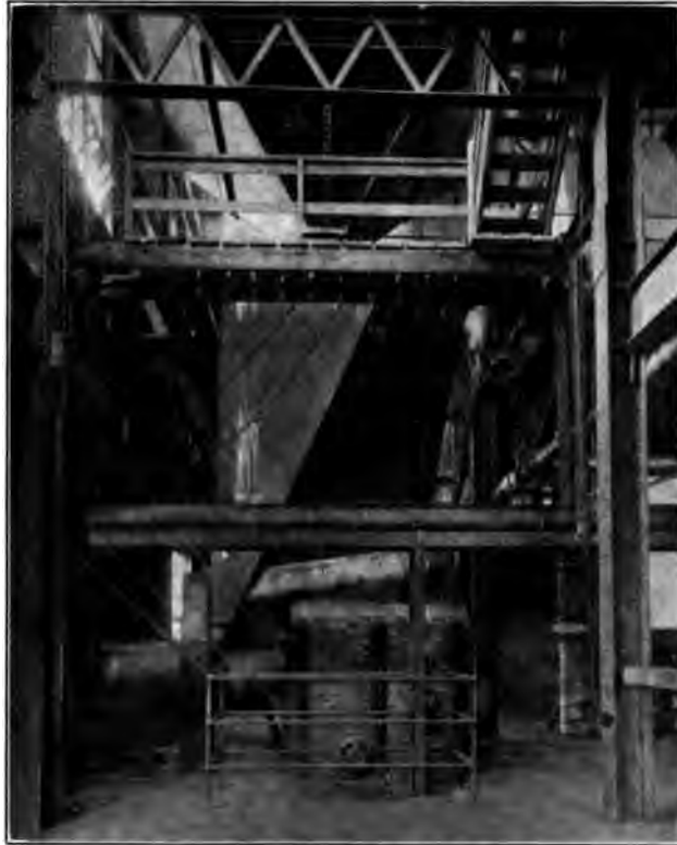
FIG. 1 Raw-Coal Storage Bin (above), with Dryer and Dryer Furnace (below), with Intermediate Connection
