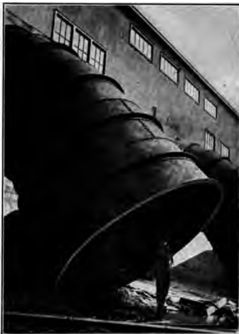
FIG. 25 76-IN. PUMP DISCHARGE, JEFFERSON-PLAQUEMINES STATION
