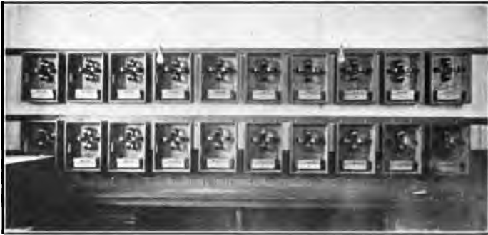
[MAGNUSSON AND BURBANK] FIG. 1—COMPLETE LINE OF TWENTY UNITS
