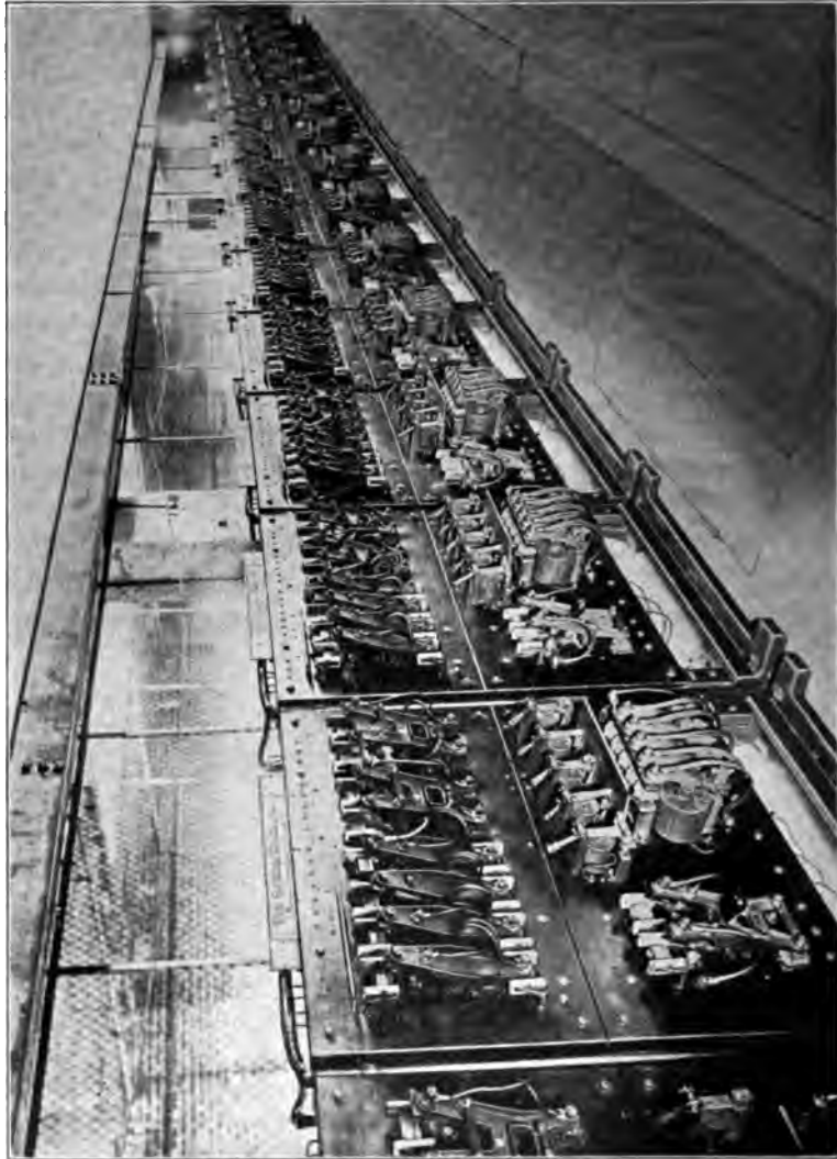
FIG. 15 A LARGE GROUP OF TRACTION ELEVATOR MACHINE CONTROLLERS IN
