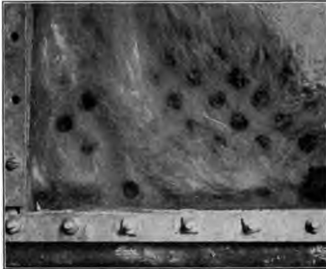
FIG. 15 SHOWING LOWER SECTION OF SAME BOILER AS IN FIG. 14; LOAD 250 PER CENT; SETTING AS IN FIG. 8b
