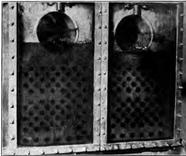
FIG. 27 SHOWING REAR HEADERS, SAME AS IN FIG. 26; LOAD 85 PER CENT; SETTING AS IN FIG. 8b
