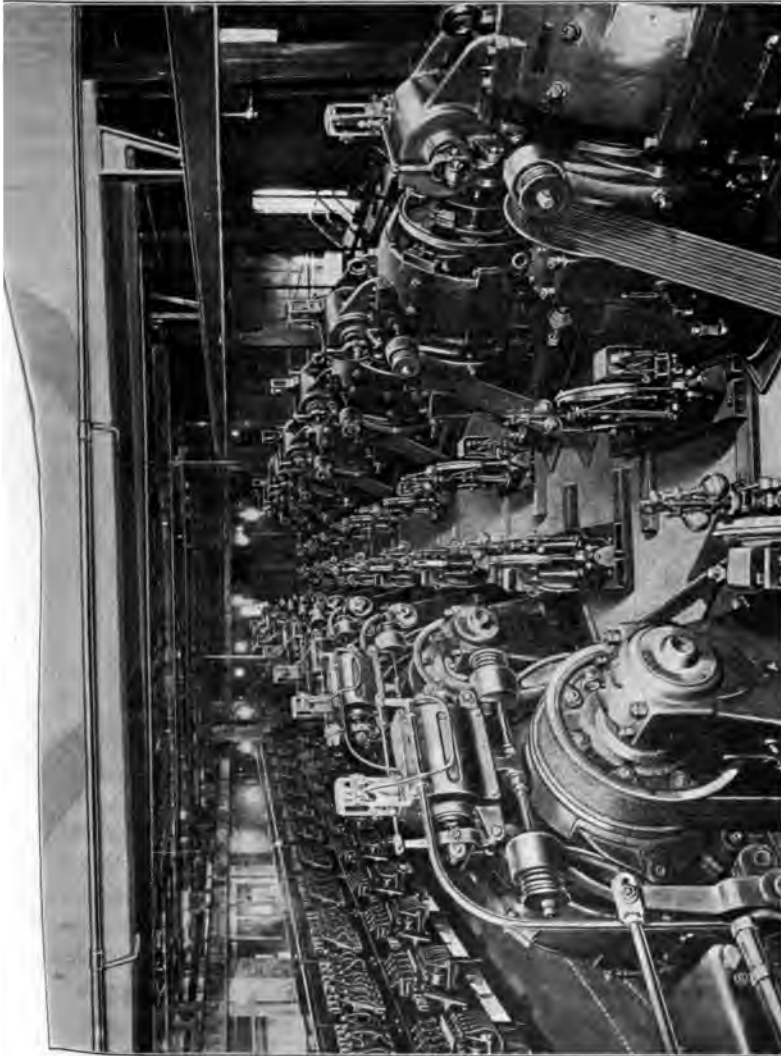
FIG. 11 TYPICAL OVERHEAD INSTALLATION OF TRACTION ELECTRIC ELEVATOR MACHINES WITH PLAIN BABBITTED BEARINGS
