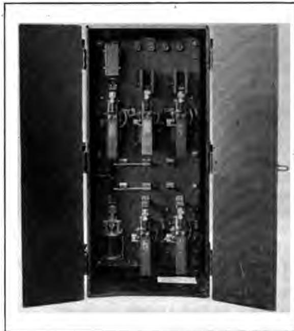
FIG. 11 WHEEL LATHE CONTROLLING PANEL. 200 AMPERE SIZE
