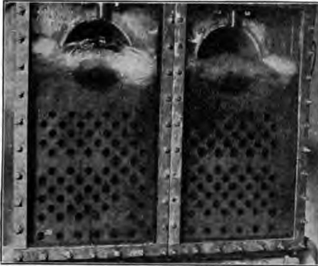
REAR HEADERS, CORRESPONDING TO DESIGN OF FIG. 11 IN FRONT; LOAD 450 PER CENT; SETTING AS IN FIG. 8b
