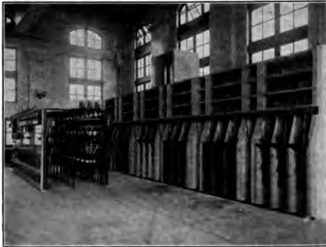
FIG. 9 SWITCHBOARD AND 11,000-VOLT COMPARTMENT FOR SUPPLYING BUSINESS DISTRICT
