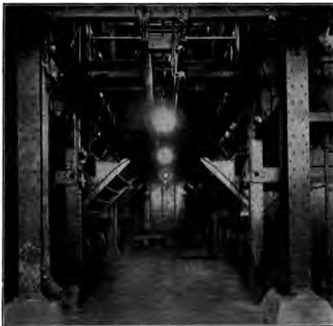
FIG. 6 VIEW IN AISLE BETWEEN BOILERS
