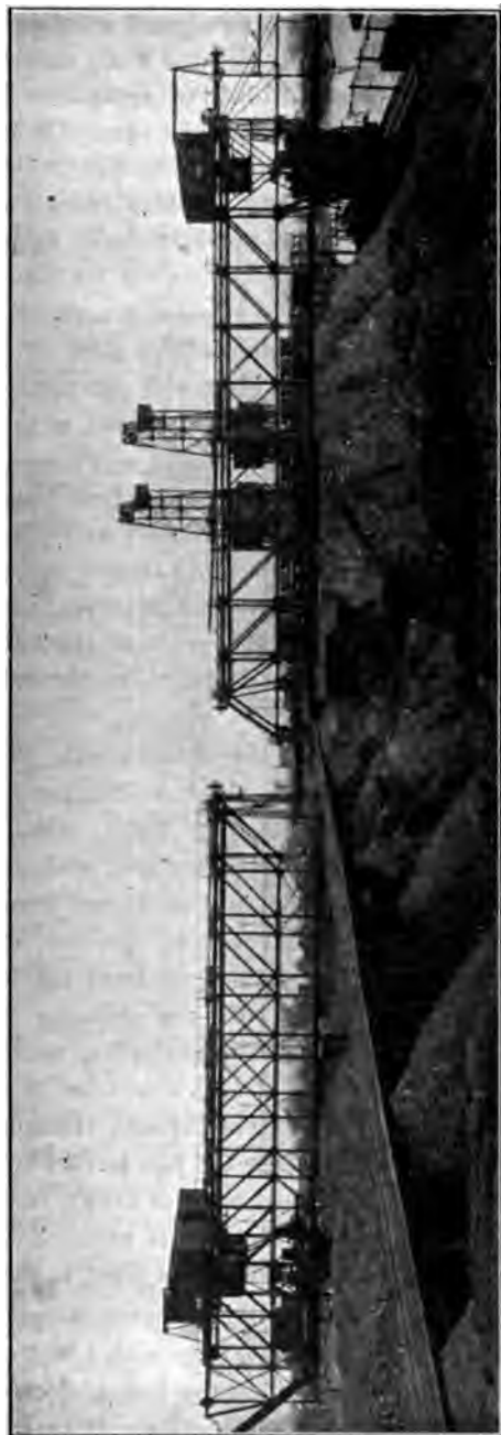
FIG. 16 MEAD HOIST TOWERS, AUTOMATIC CARS, CABLE RAILWAY AND BRIDGES, MILWAUKEE WESTERN FUEL COMPANY'S WASHINGTON STREET DOCK, MILWAUKEE, WIS.
