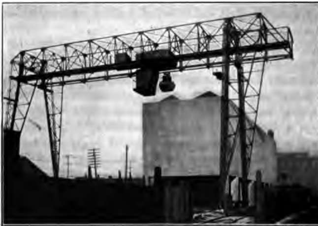
FIG. 41 MCMYLER MECHANICAL PLANT FOR RETAIL YARD, CLEVELAND AND PITTSBURGH COAL COMPANY'S RETAIL YARD, CLEVELAND, OHIO
