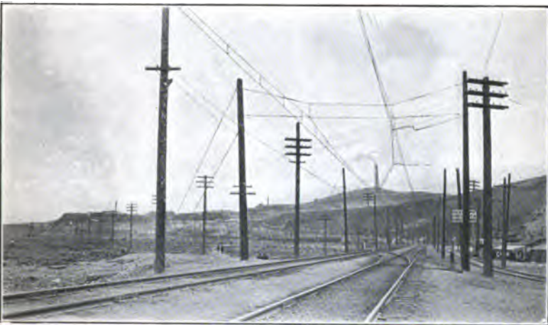
FIG. 14—DOUBLE TRACK SPAN CONSTRUCTION ON MAIN LINE AND GENERAL VIEW OF SMELTER HILL FROM WEST OF EAST ANACONDA YARDS
