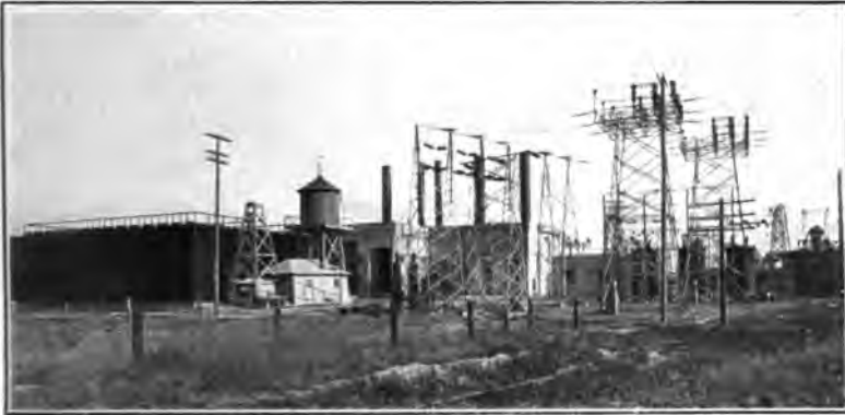
[THOMAS] FIG. 66—SOUTHERN SIERRAS POWER CO. SAN BERNARDINO OUTDOOR TRANSFORMER STATION
