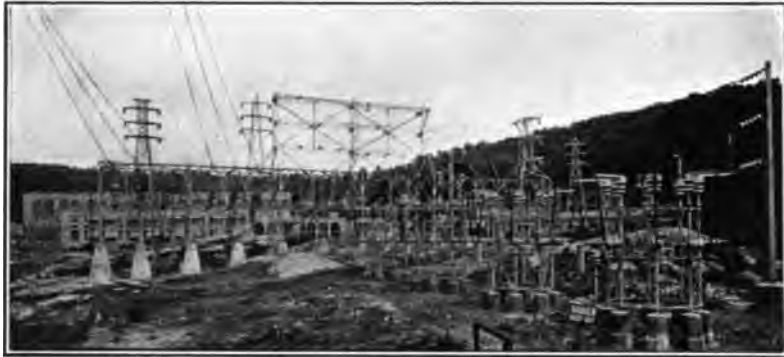
[THOMAS] FIG. 72—PENNSYLVANIA WATER AND POWER CO. NICHOLSON'S LIGHTNING ARRESTERS
