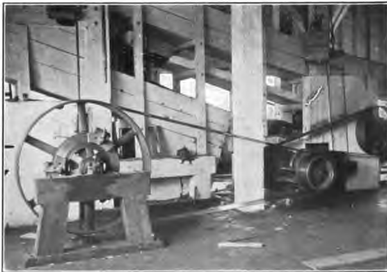
FIG. 34—BACK-GEARED MOTOR BELTED TO BURNER CONVEYER [WHITNEY]
