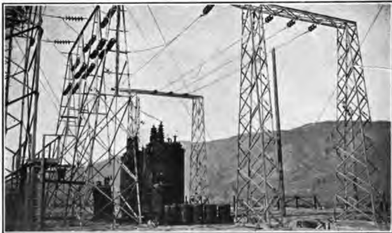
[THOMAS] FIG. 69—SOUTHERN SIERRAS POWER CO. LONE PINE SUBSTATION
