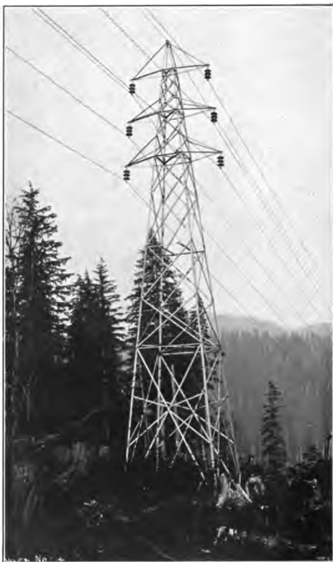
[NIMS] FIG. 2—STANDARD STEEL TOWER WITH GROUND WIRE ON APEX
