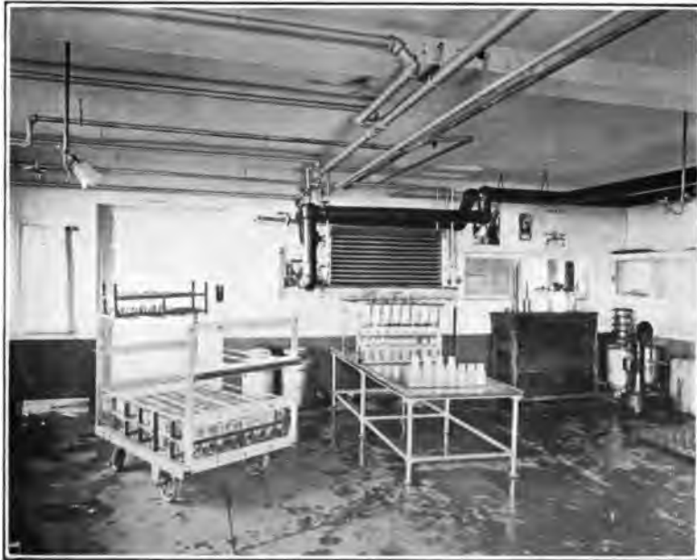
[BATES] FIG. 20—MILK COOLER AND AERATOR CONNECTED WITH INSULATED BRINE LINES RUNNING FROM BRINE TANK OF THE ELECTRICALLY-DRIVEN REFRIGERATING PLANT SHOWN IN FIG. 19.
