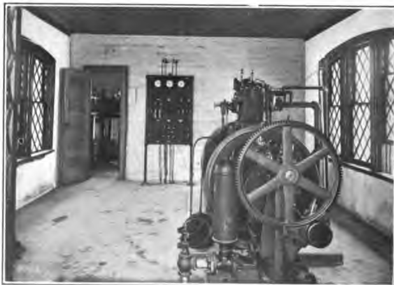
FIG. 33—AN IDEAL PUMPING PLANT FOR FIRE PROTECTION. [BATES]
