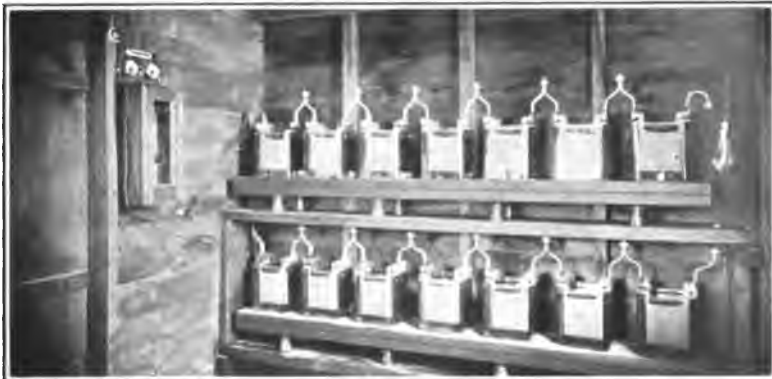
FIG. 31—STORAGE BATTERY IN ADJOINING BARN, ACCUMULATES [BATES] ENERGY GIVEN BY DYNAMO WHEN RUNNING, AND STORES IT FOR USE WHEN LIGHTS ARE TURNED ON.
