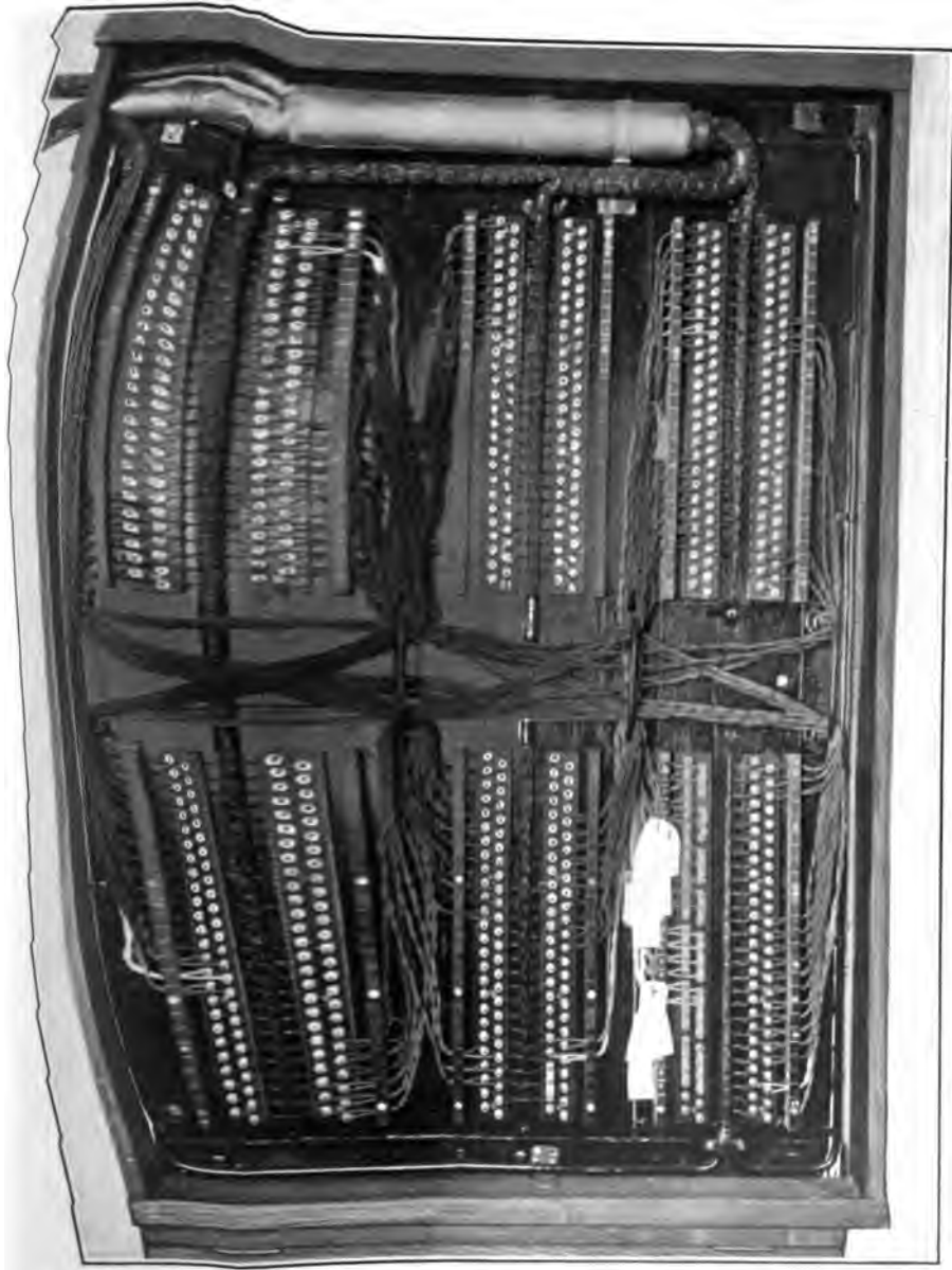
FIG. 1—MAIN TERMINAL BOX, CAPACITY FOR TERMINATING [RHODES] 312 PAIRS OF WIRES.
