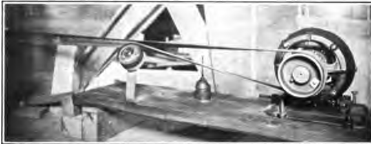
FIG. 30—THE DYNAMO HAS A CAPACITY OF 0.21 KW. [BATES] It is set on the second floor of the mill, and is driven by a quarter-turned belt from a pulley on the vertical shaft of the windpower.
