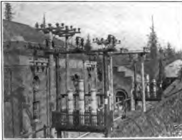
Switching and lightning arresters at Snoqualmie Falls
