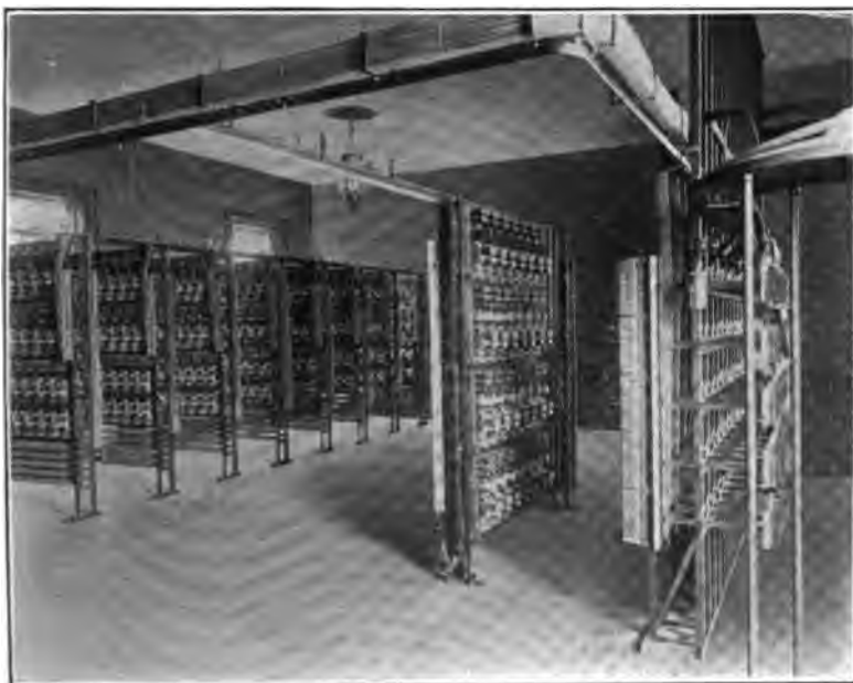
FIG. 6.—Automanual switch-room—Warren, Ohio., showing main frame and secondary switch panel
