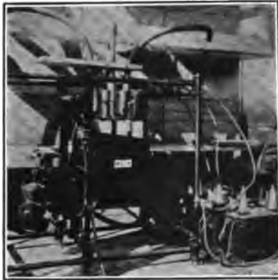
FIG. 4.—Solenoid-operated oil circuit breaker used for throwing on short circuits
