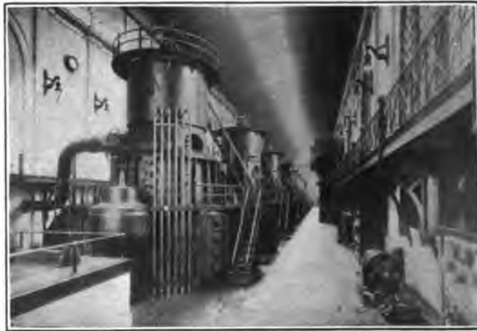
FIG. 1. —Interior of Fisk street station, Commonwealth Edison Company
