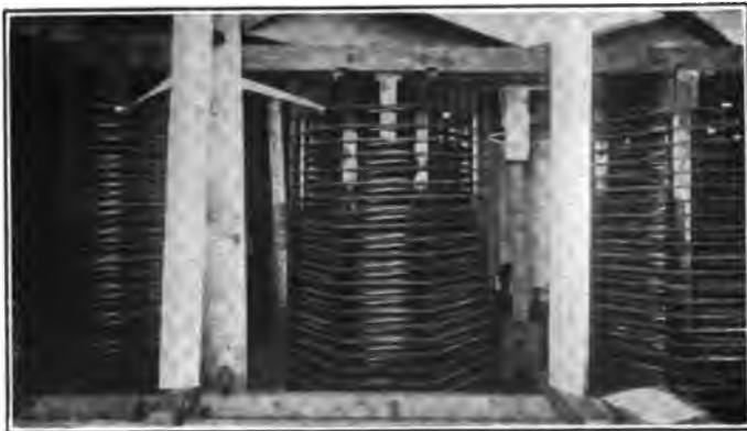
FIG. 5.—Flashlight of generator current-limiting reactances during test No. 27
