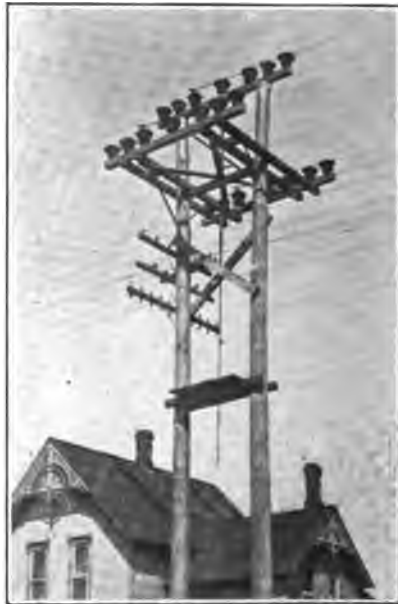
Standard pole switch. (60,000 volts)
