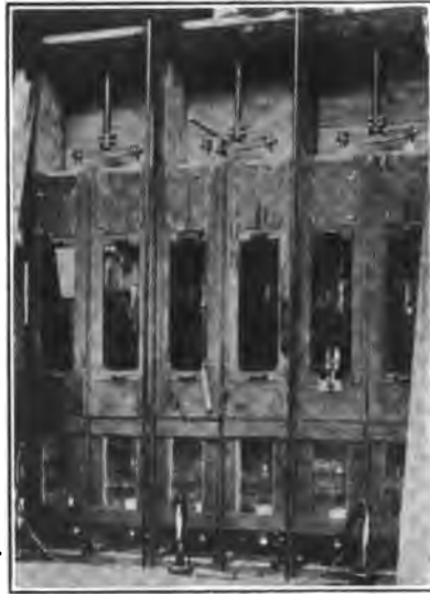
FIG. 7.—Type F form H-6 oil circuit breaker during test No. 27
