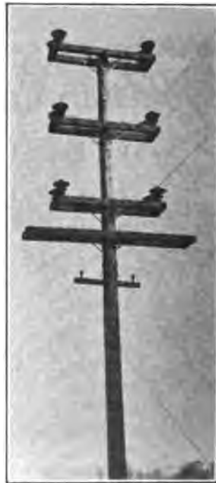
Pole-top construction where two lines are on the same pole, showing guard wires over railroad. (60,000 volts)
