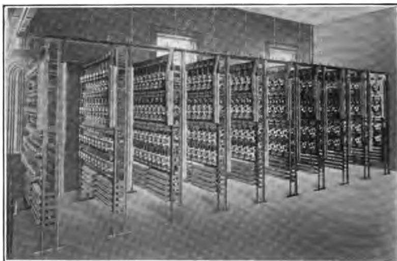
FIG. 7.—Automanual connecting-switch racks—Warren, Ohio., showing arrangement of 100-line units
