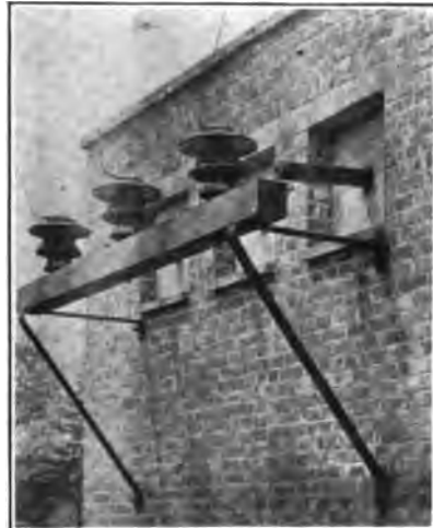
Entrance tubes at substations. (60,000 volts)
