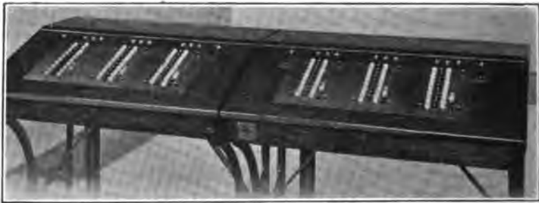
FIG. 1.—Automanual operating equipment—Ashtabula Harbor
