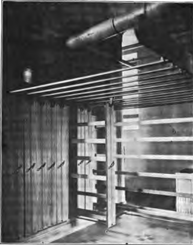
FIG. 4—Dry room, showing clothes racks and air flue
