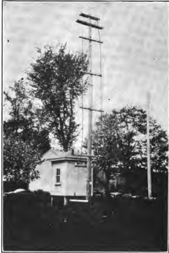
FIG. 4.—Presumpscot Electric Co. View of Eel Weir half-way line lightning arrester house
