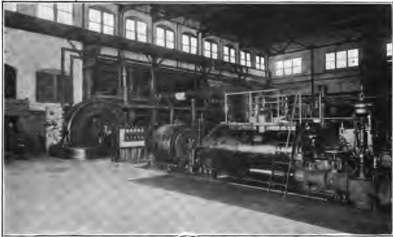
FIG. 1 —Non-Synchronous generator installed at a copper-smelting and rolling mill.
