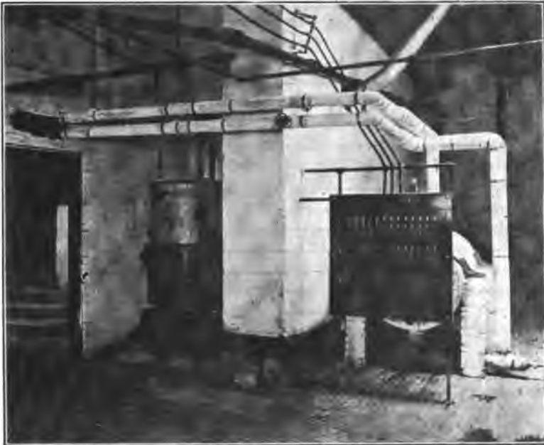
FIG. 1.—Fuel and electric hot water heaters
