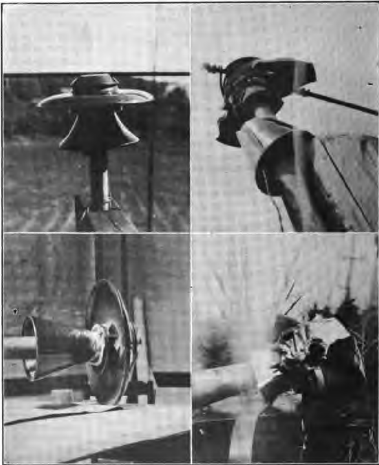
Shattered 8/18/07, pole 1341 Punctured 6/29/07, pole 1474
