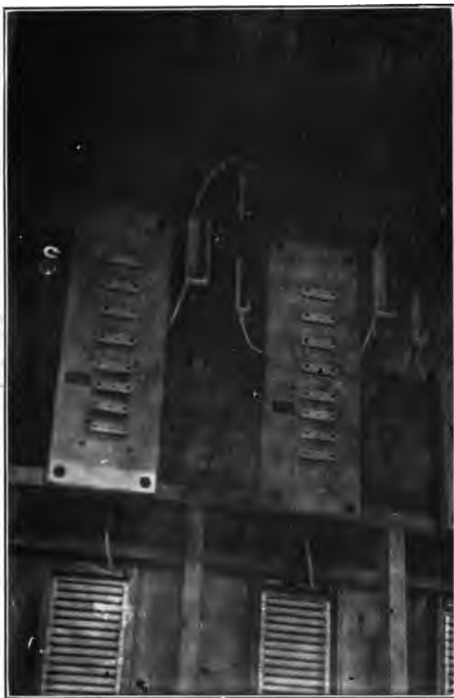
FIG. 5.—Presumpscot Electric Co. Interior of Eel Weir half-way line lightning arrester house
