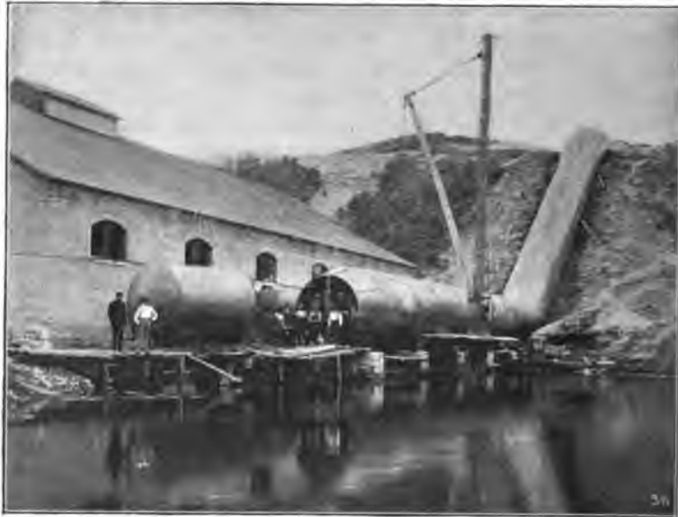
FIG. 7.—12 feet Steel Penstock.
