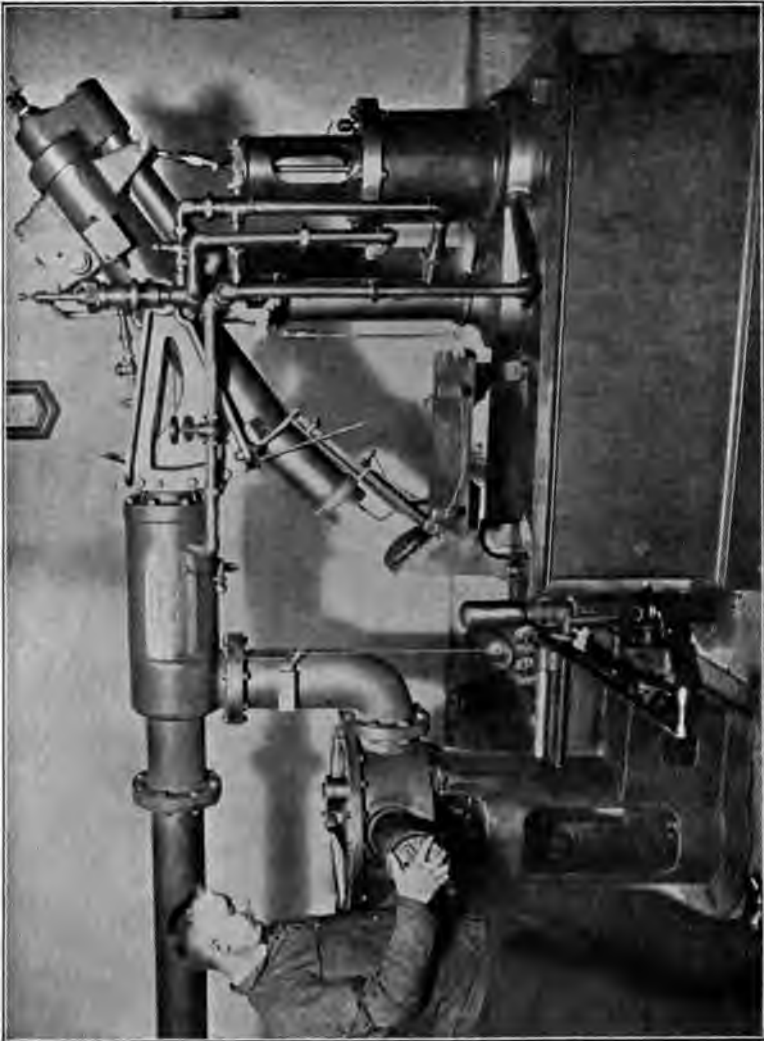
FIG. 122.—SIX-INCH TUBE SENDING AND RECEIVING APPARATUS AT THE BOURSE, PHILADELPHIA.
