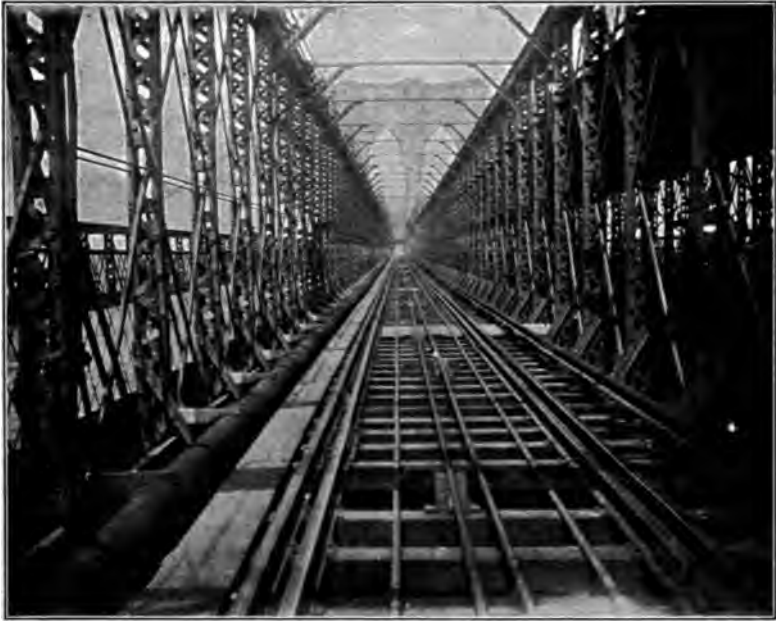
FIG. 136.—PNEUMATIC TUBES ON THE NEW YORK AND BROOKLYN BRIDGE.
