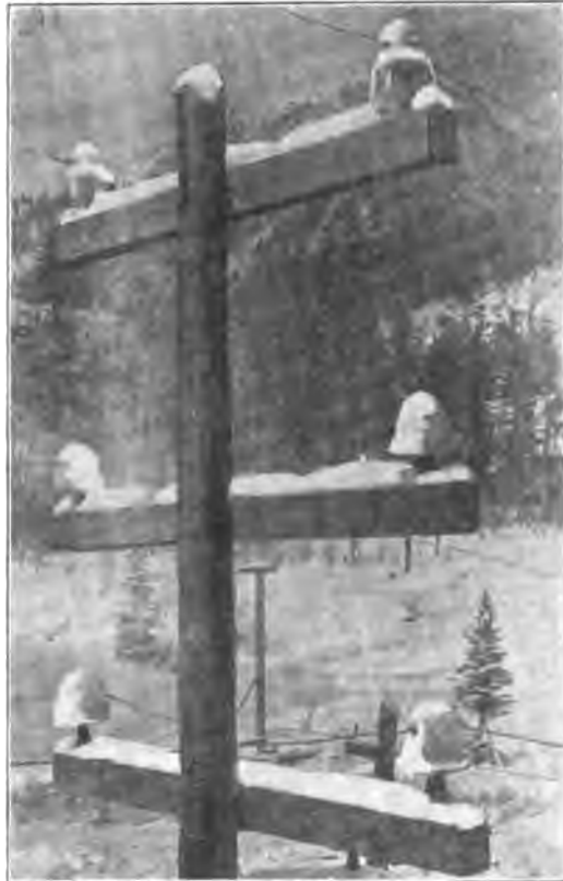
FIG. 4.—50,000 Volts on Large Glass Insulators (Upper Cross-arm) and on Porcelain Insulators (Lower Cross-arm.)
