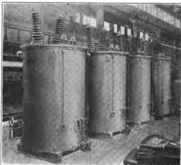
THE FOUR 23,600-KV-A. TRANSFORMERS
