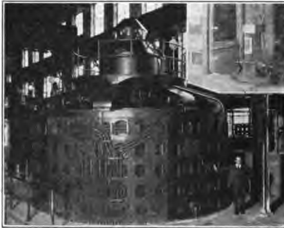
FIG. 2—EARLIEST AND LATEST COMMERCIAL GENERATORS TO OPERATE BY NIAGARA POWER
