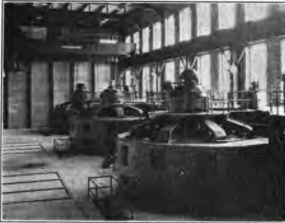
FIG. 21—INTERIOR OF STATION NO. 3 EXTENSION AFTER PLACING OF VENTILATING HOUSINGS AROUND GENERATORS
