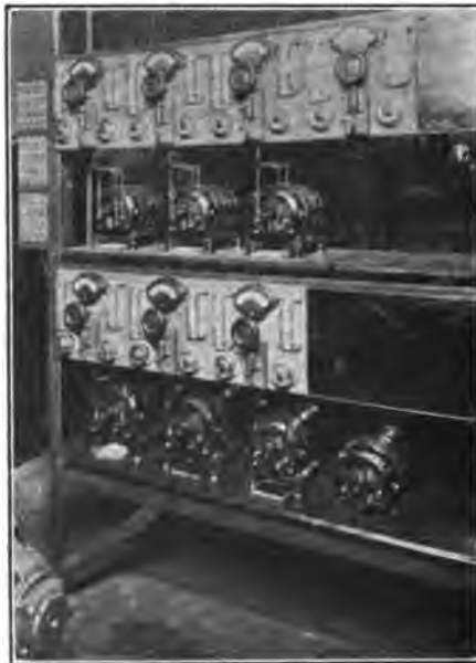
FIG. 15—UNIT TYPE POWER SWITCHBOARDS FOR SELECTOR TELEPHONE CIRCUITS
