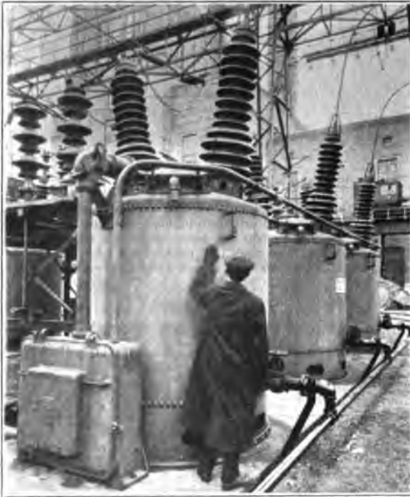
A 132,000-VOLT, 400-AMPERE CIRCUIT BREAKER
