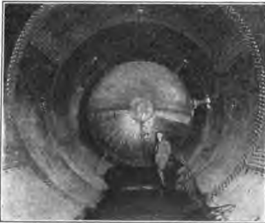
FIG. 17—UPSTREAM END OF JOHNSON VALVE INSIDE OF PENSTOCK
