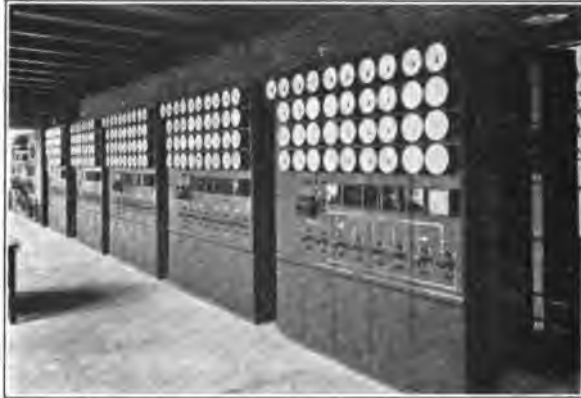
FIG. 32—SWITCHBOARD AT ECHOTA SUBSTATION
