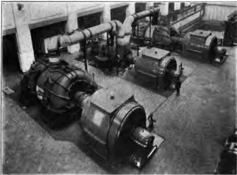
GENERAL VIEW OF 60,000-KW. UNIT
