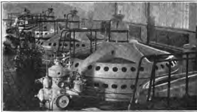
FIG. 11—FIVE VERTICAL A-C. GENERATORS—THRUST BEARINGS CARRIED ON UPPER HOUSINGS
