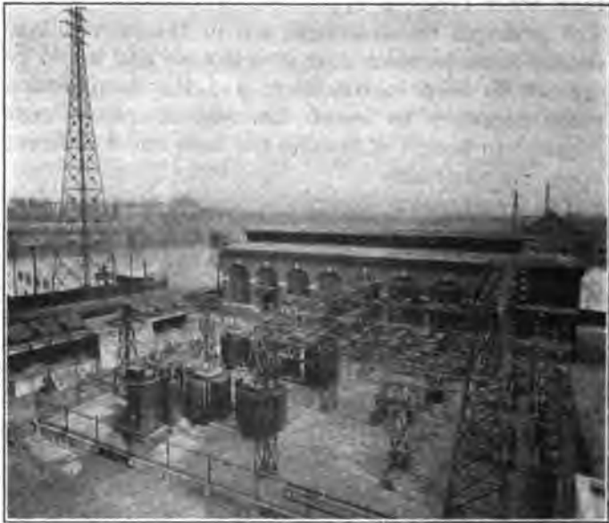
FIG. 6—GENERAL VIEW OF THE OUTDOOR SUBSTATION IN WHICH THE REGULATORS ARE INSTALLED
