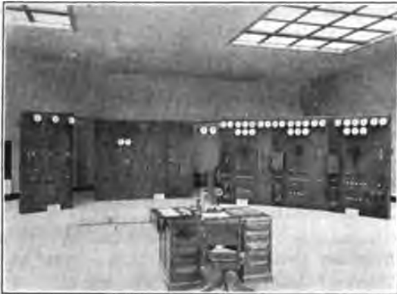
FIG. 23—CONTROL ROOM SHOWING PANELS FOR CONTROL OF 100,000 H. P. STATION NO. 3 EXTENSION
