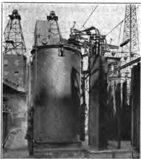
FIG. 7—CLOSE-UP VIEW OF ONE OF THE 1750 KV-A. INDUCTION REGULATORS
