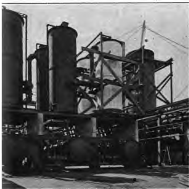
PHLEGMATORS WITH HEAT EXCHANGERS UNDERNEATH
