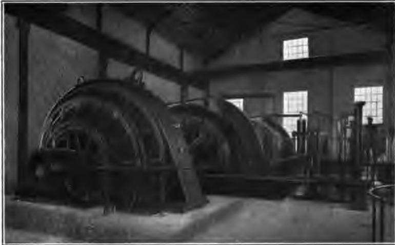
FIG. 1—VIEW OF HOIST MOTOR
