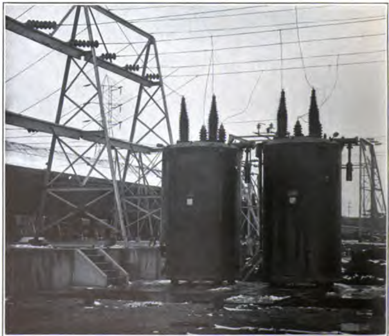
[GREEN] FIG. 4—OUTDOOR INSTALLATION OF 100,000-VOLT TRANSFORMERS
