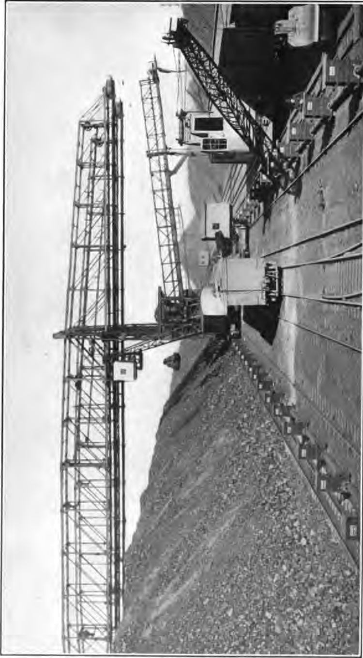
FIG. 2—BRIDGE TRAMWAY Showing locomotive cranes, box-car loaders, screening towers and current posts [EYERSON AND CRANE]
