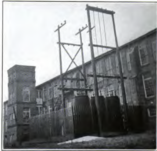
[GREEN] FIG. 3—OUTDOOR INSTALLATION OF 100,000-VOLT TRANSFORMERS
