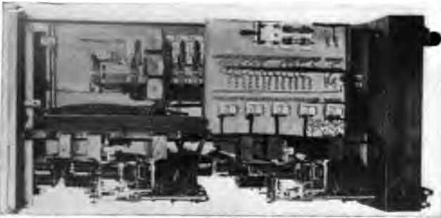
[DEAKIN] FIG. 6C—SIDE ELEVATION OF 25-LINE SWITCHBOARD Doors removed, showing power panel, terminal strips and miscellaneous relays
