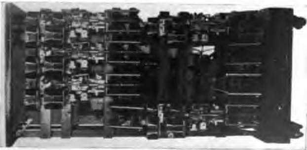
[DEAKIN] FIG. 6B—REAR ELEVATION OF 25-LINE SWITCHBOARD Doors removed, showing "mechanical operators," connectors and banks
