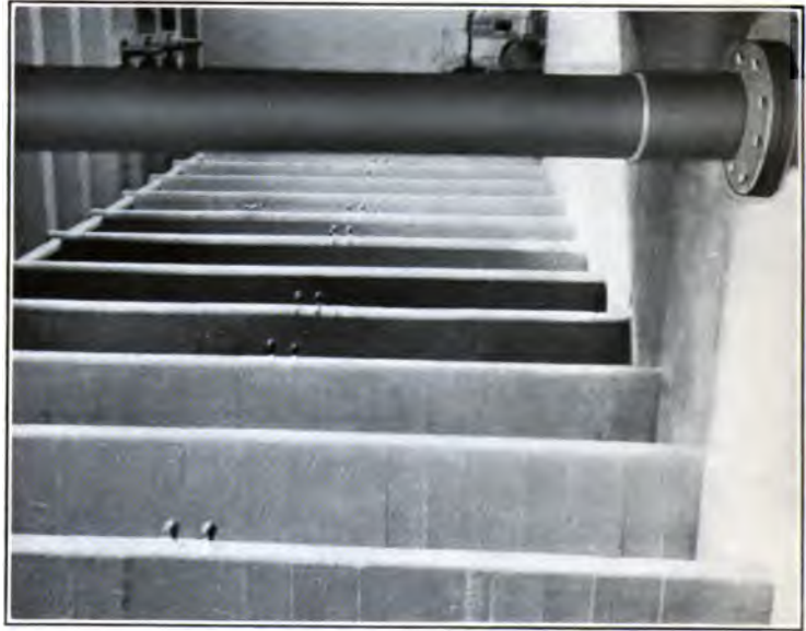
[GREEN] FIG. 8—COMPARTMENT TYPE OF INSTALLATION—HIGH-VOLTAGE BUS COMPARTMENTS
