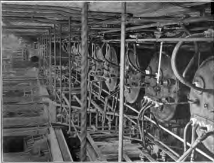
[GREEN] FIG. 5—OPEN TYPE OF TRANSFORMER INSTALLATION IN CLOSE QUARTERS
