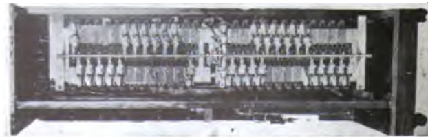
[DEAKIN] FIG. 7A—FRONT ELEVATION OF 50-LINE SWITCHBOARD Doors removed, showing a partial equipment of line switches
