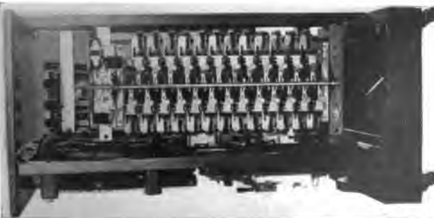
[DEAKIN] FIG. 6A—FRONT ELEVATION OF 25-LINE SWITCHBOARD Door removed, showing line switches
