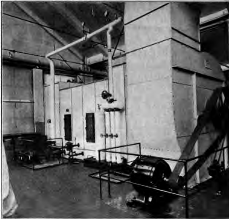
FIG. 6 GENERAL VIEW OF HUMIDIFIER
