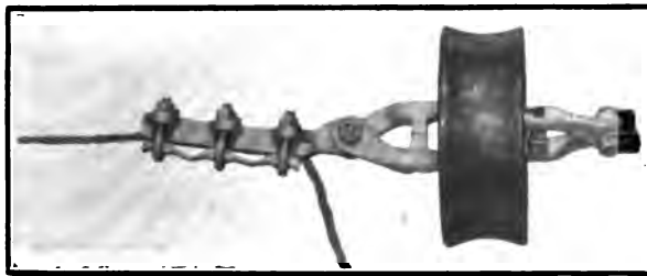
FIG. 10.—25,000-volt link strain insulator
