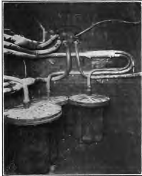
FIG. 3.—Underground man-hole containing loading coils
