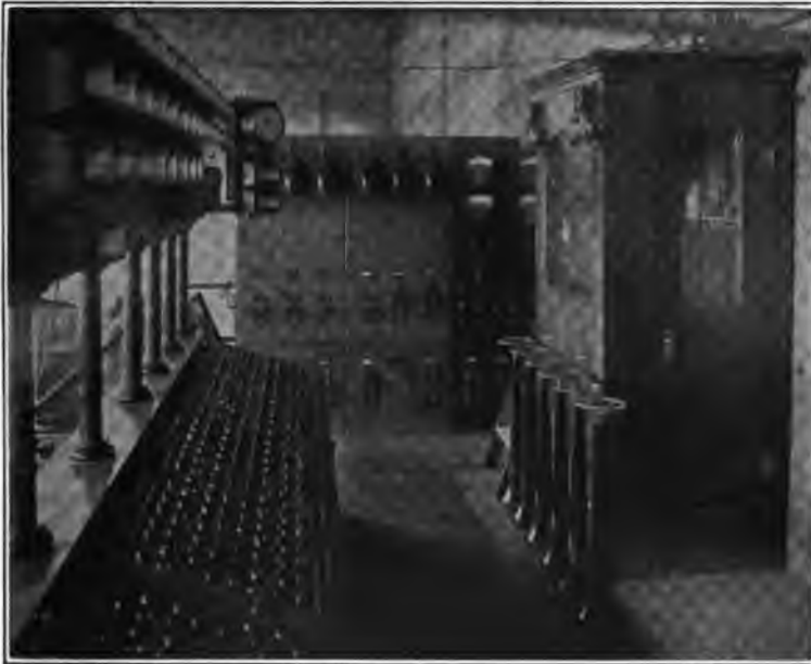
FIG. 23.—Switchboard, Roosevelt power house.
