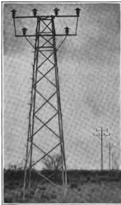
FIG. 25.—Roosevelt-Phoenix transmission line in the valley.
