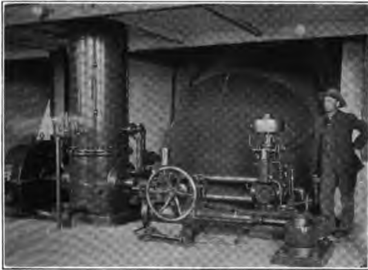
FIG. 7.—Oil pump and governor, Minidoka power house.
