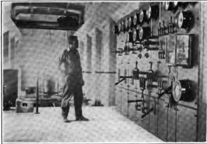
FIG. 14.—Switchboard pumping station No. 2, Minidoka project.
