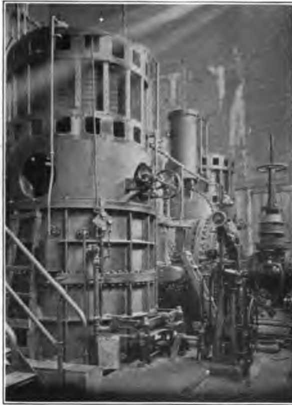
FIG. 22.—Interior, Roosevelt power house, before completion, showing vertical turbines and generators.
