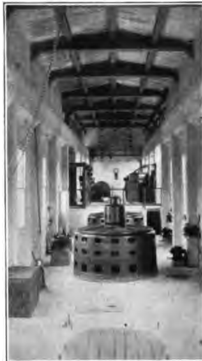
FIG. 12.—Interior Pumping station No. 2 Minidoka project
