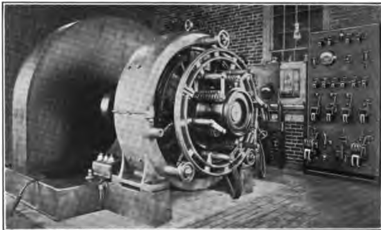
FIG. 1.—Flywheel generator set
