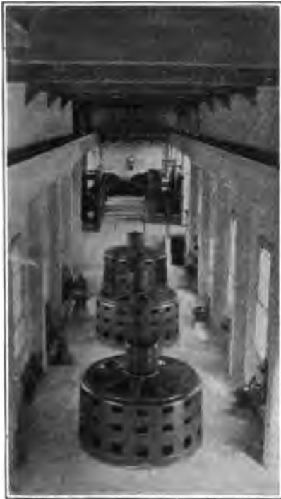
FIG. 11.—Interior pumping station No. 1, Minidoka project
