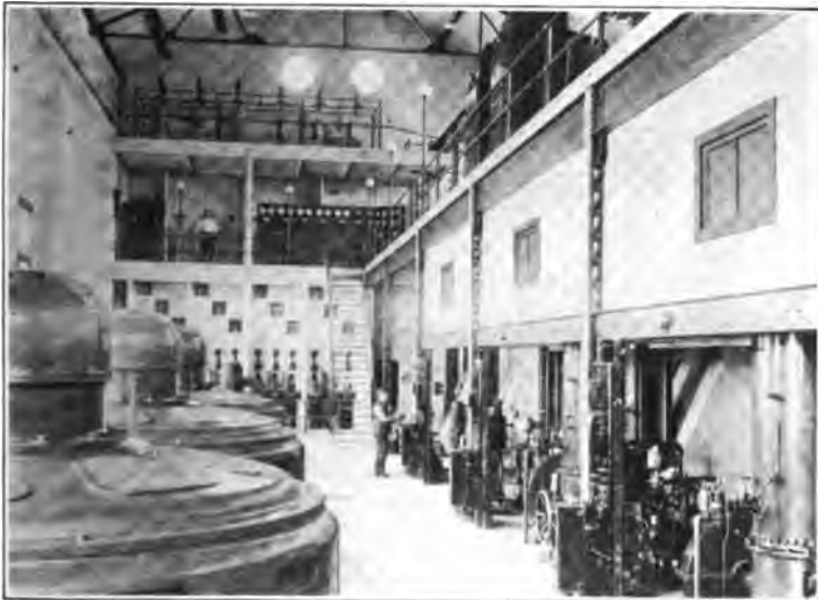
FIG. 5.—Interior, Minidoka power house.
