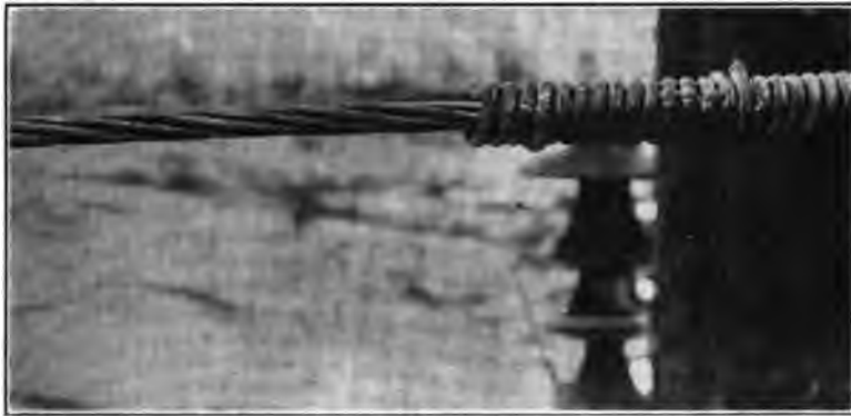
FIG. 9.—214,000 cir. mils aluminum cable burned by three applications of a 1200-ampere arc
