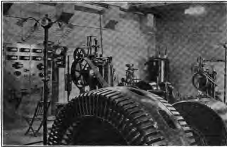
Cottonwood power house—two 750-kw. generators—power all utilized for construction work
