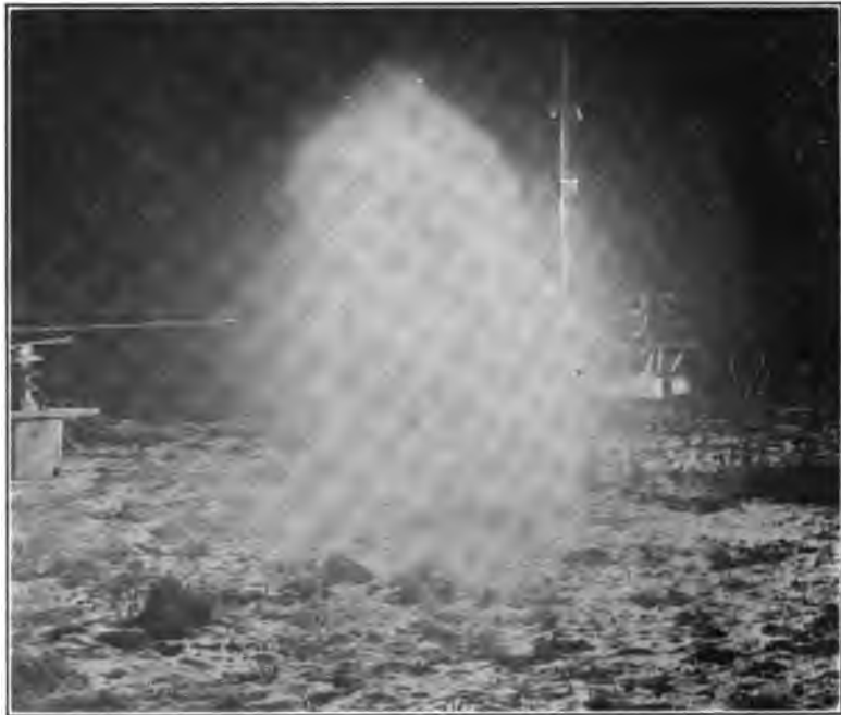
FIG. 8.—Night photograph of a 30,000-kw. 1200-ampere arc on an insulator equipped with arcing rings
