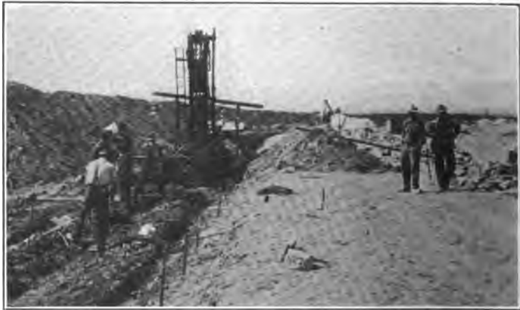
Electric shovel on open conduit; Mojave Valley
