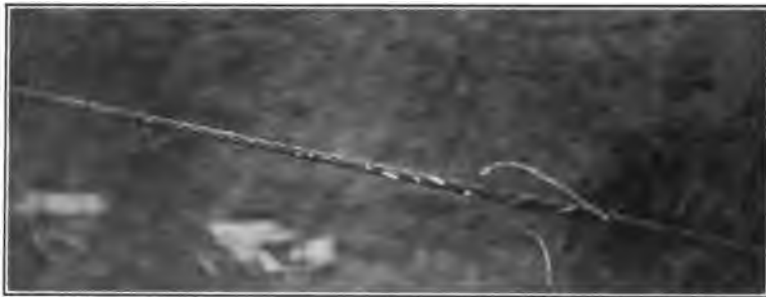
FIG. 10.—214,000 cir. mils aluminum cable burned in service by a short-circuit arc from six 10,000-kw. generators
