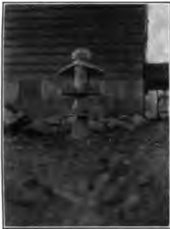
FIG. 15.—Insulator injured in head-piece by power arc. No upper arcing ring was installed
