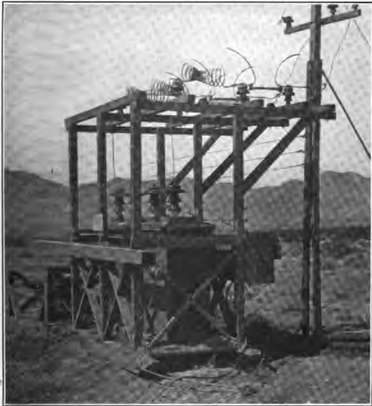
33,000-volt portable substation—outdoor type transformers
