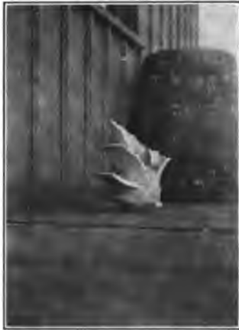
FIG. 13.—Four-part insulator destroyed by power arc. The only insulator disabled on the reinsulated lines 1909
