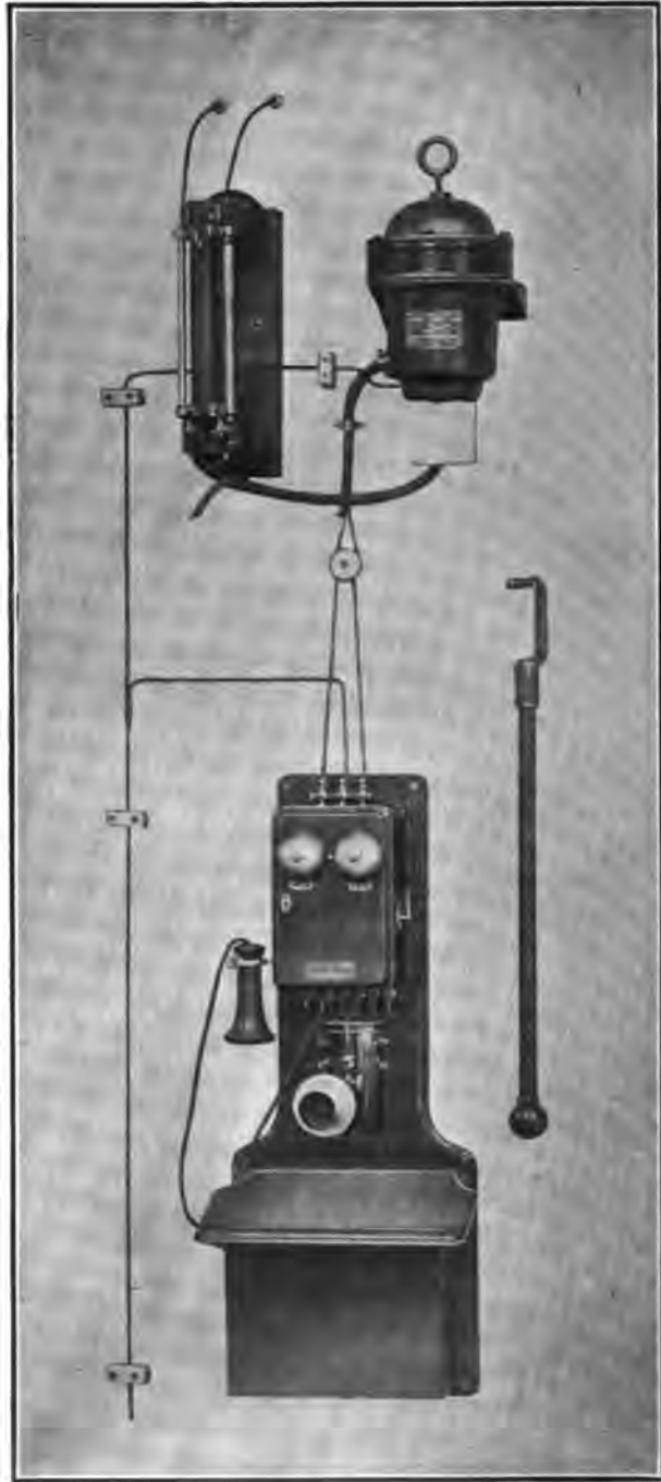
FIG. 12—Installation of telephone, with Y-109 insulating transformer and combination fuse lightning-arrester and disconnecting switch.
