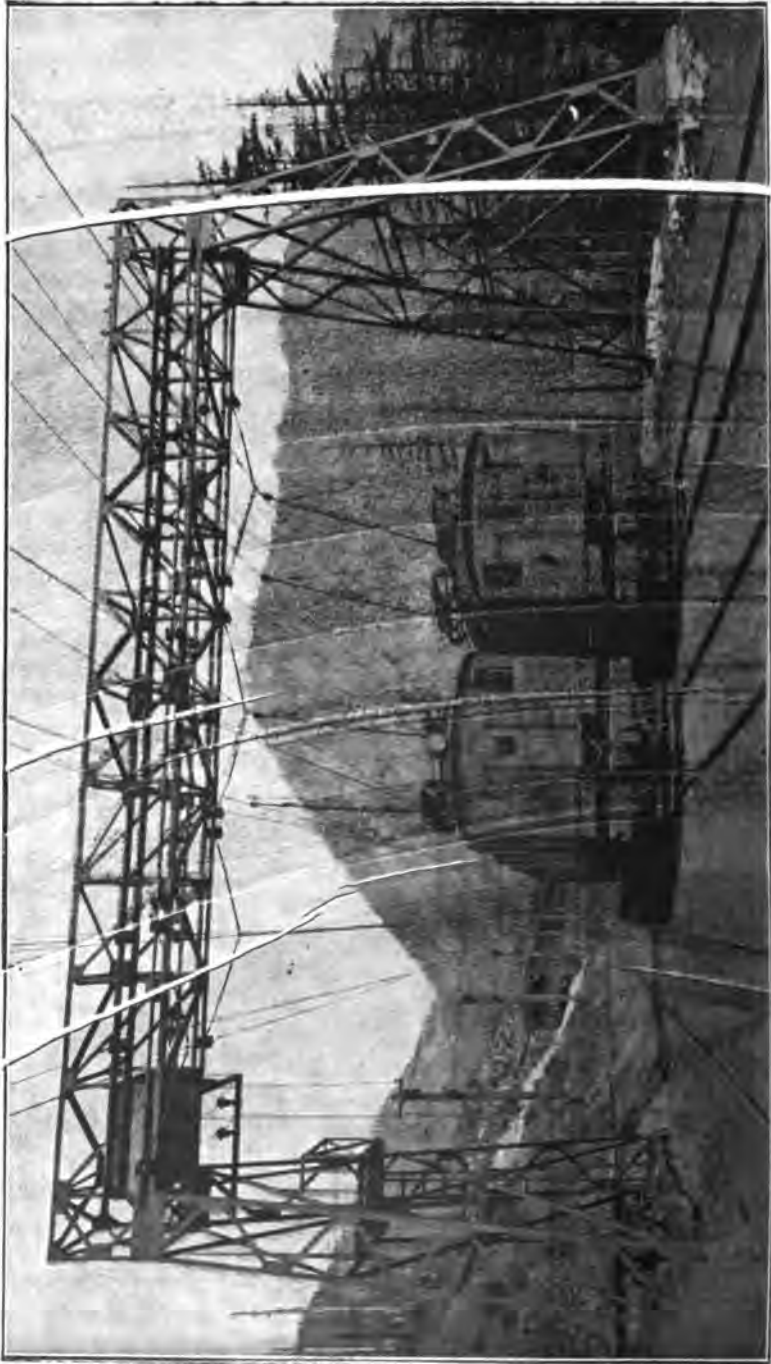
FIG. 14.—Anchor bridge in Wellington yard, showing three tracks electrified
