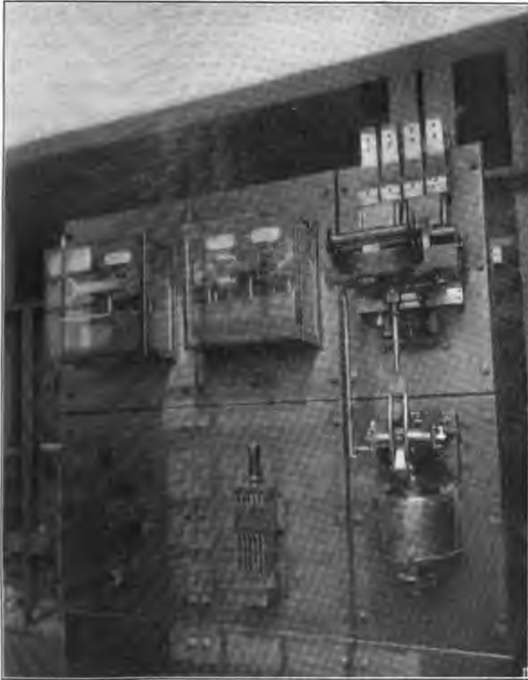
FIG. 8.—Battery switchboard, negative side, Indiana Steel Co., Gary, Ind.
