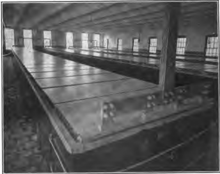
FIG. 1.—Battery room second floor diagonal view, Indiana Steel Co., Gary, Ind.
