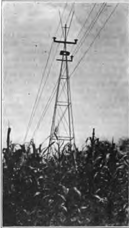
FIG. 2—Showing first change. Top insulator lowered, grounded cable in place, and lightning-rods left in position
