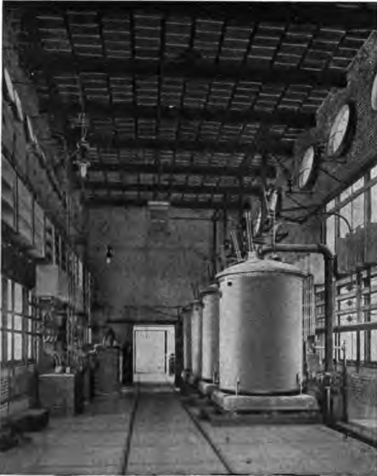
FIG. 33—Transformer room, Lockport sub-station
