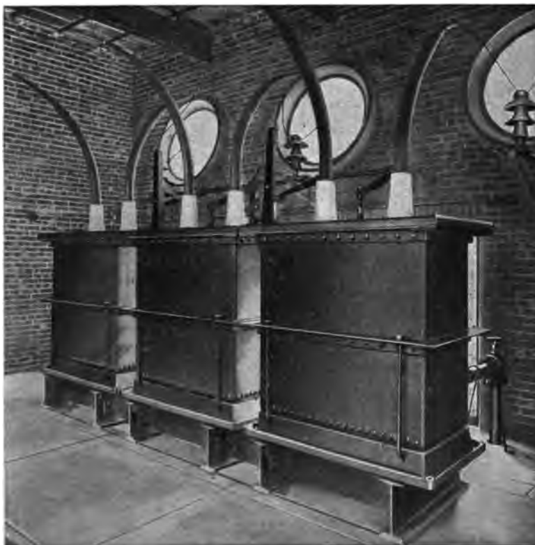
Fig. 35—60,000-volt oil-switch and circuit-breaker, electrically operated
