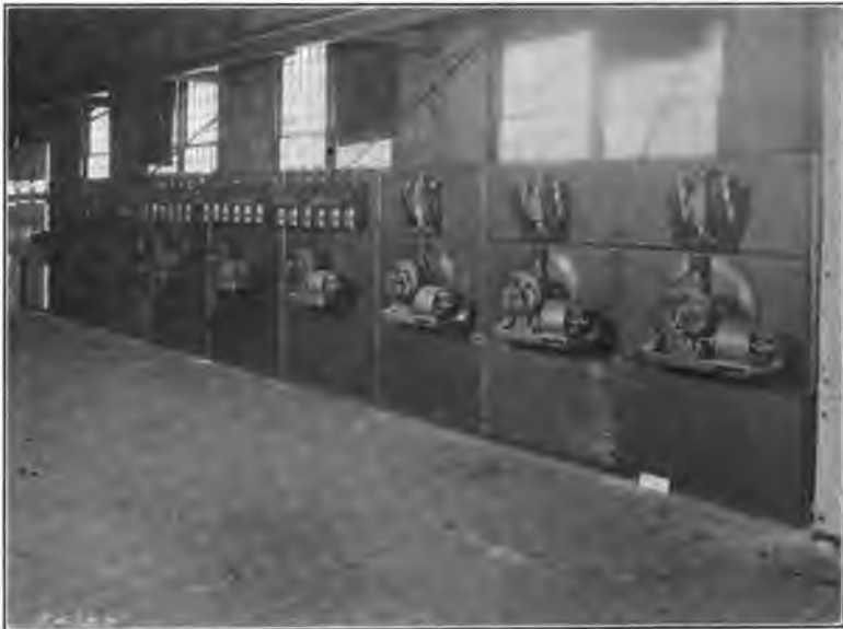
FIG. 2—Switchboard for exciter and field control for 88,000-volt plant.
