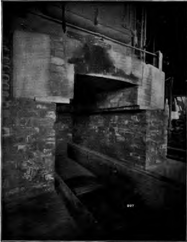
FIG. 129.—FURNACE FITTED TO RECEIVE BABCOCK & WILCOX STOKER.
