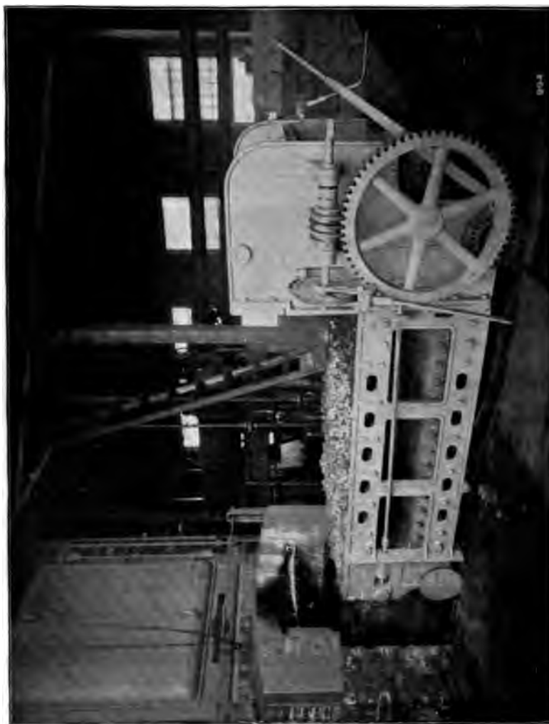
FIG. 127.—BABCOCK & WILCOX STOKER REMOVED FROM FURNACE.
